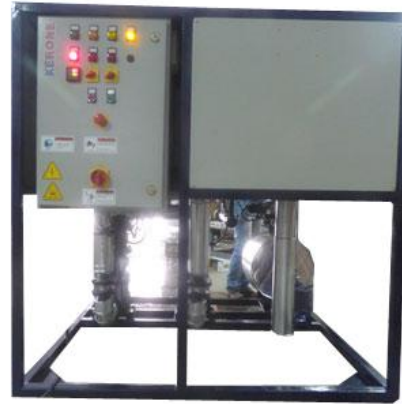
Hot Water Systems
